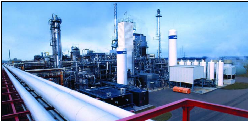
Linde pipelines carrying hydrogen and carbon monoxide
